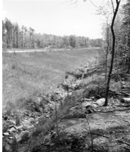
Fig. 6-3 Canal al borde de una carretera. (AASHTO, 3.5.2 Permanent Erosion and Sediment Control Measures; Chapter 3 - Erosion and Sediment Control in Highway Construction, 2006)
