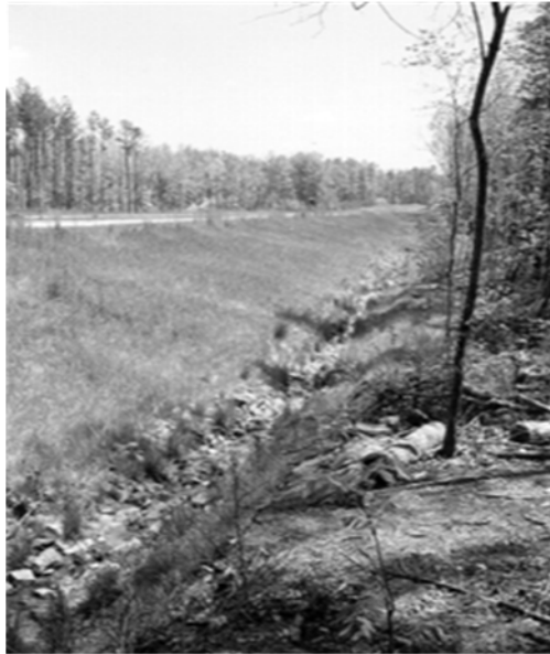
Fig. 6- 3 Canal on the edge of a road. (AASHTO, 3.5.2 Permanent Erosion and Sediment Control Measures; Chapter 3 - Erosion and Sediment Control in Highway Construction, 2006)
