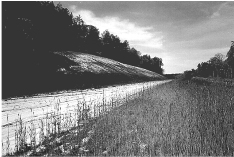
Fig. 6-1 Example of embankments of each side of the road. (AASHTO, 3.5.2 Permanent Erosion and Sediment Control Measures; Chapter 3 - Erosion and Sediment Control in Highway Construction, 2006)
