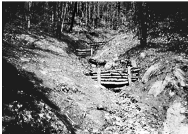
Fig. 6-4 Control structures in Wood canals. Extracted from (AASHTO, 3.5.2 Permanent Erosion and Sediment Control Measures; Chapter 3 - Erosion and Sediment Control in Highway Construction, 2006)
