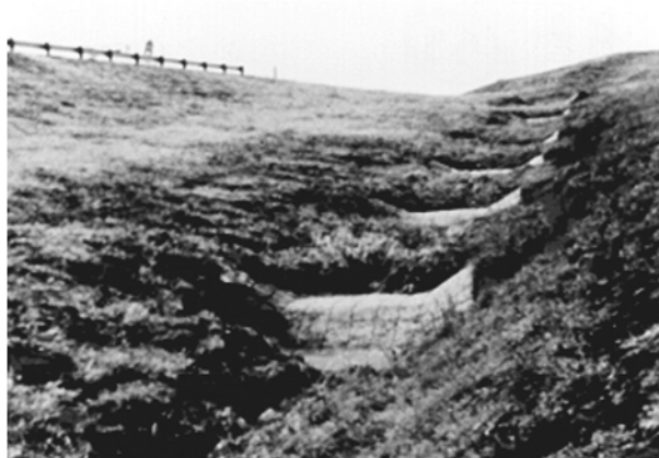
Fig. 6-5 Control structures in hydraulic concrete canals. Extracted from (AASHTO, 3.5.2 Permanent Erosion and Sediment Control Measures; Chapter 3 - Erosion and Sediment Control in Highway Construction, 2006)
